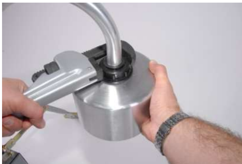
PIPE WRENCH TIGHTENING NUT ONTO RUBBER WASHER (NOTE: LEFT-HANDED COUNTER-CLOCKWISE THREAD ON NUT )
