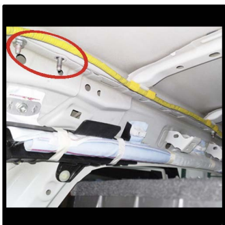
The bolts holding the roof rails in are now exposed and the nuts can now be removed.
