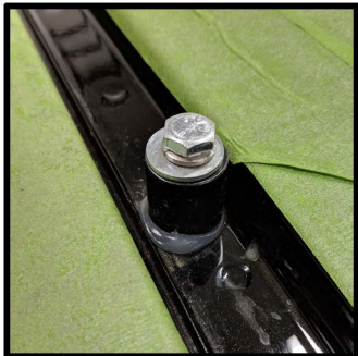
Apply more silicone to insure a water tight seal and place the spacer on the roof.
