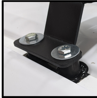
Then place the mounting feet down and bolt them to the roof
