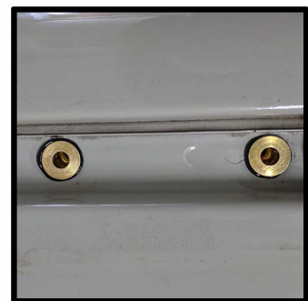
Plusnuts in roof, one plus nut is not used for mounting and comes with a washer & 1" bolt to seal it
