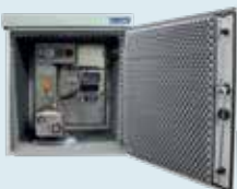
L metal external cabinet
