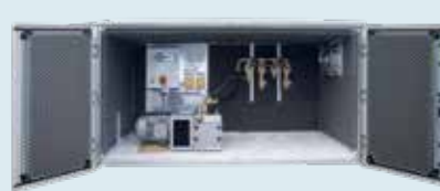
Concrete external cabinet
