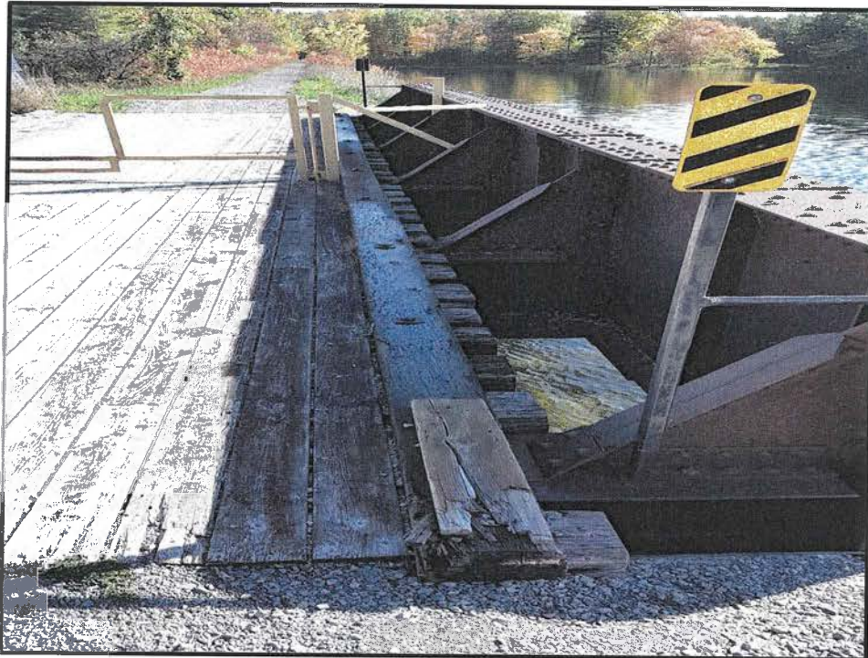
Deck to Truss Gap (To Be Filled or Guarded with Rail)
