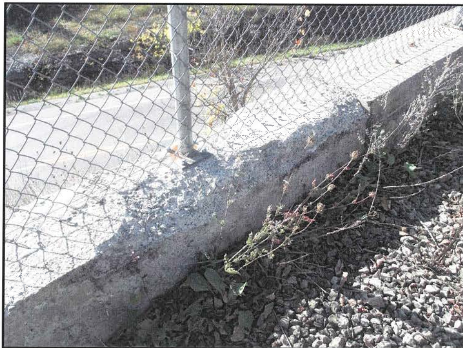
Scaling on Expose Top Section of NE Wingwall
