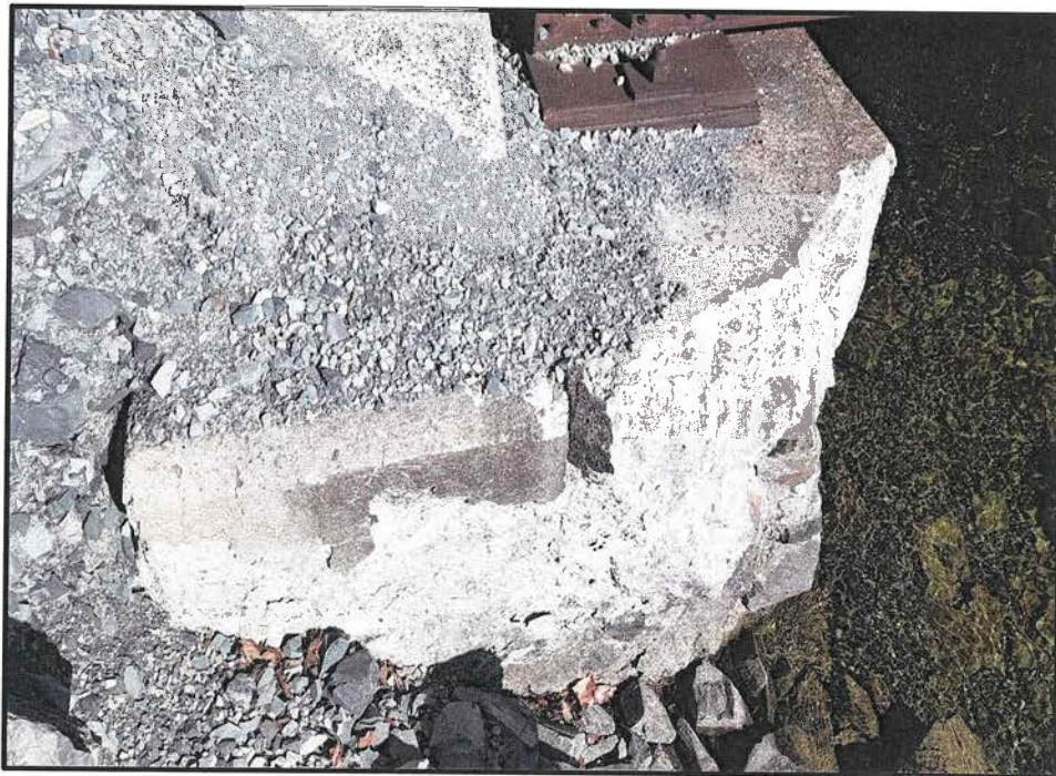
Severe Cracking and Spall at SW Abutment Wall
