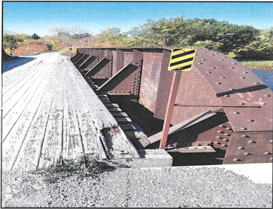
Damaged NE Corner of Timber Curb
