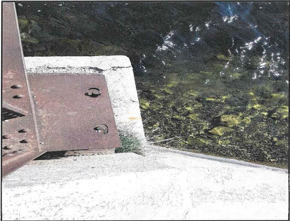
Severe Cracking on SW Bearing Seat
