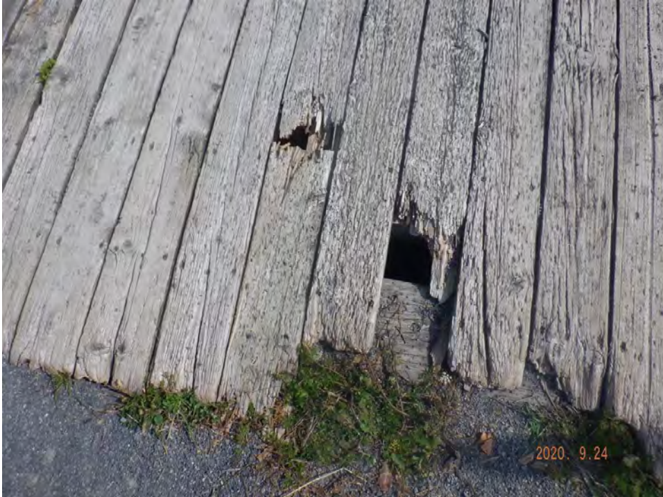
Rot in west deck end
