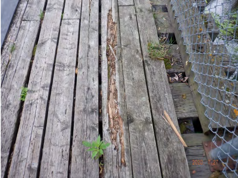
Rot in deck boards
