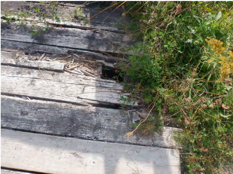
Rot in deck surface
