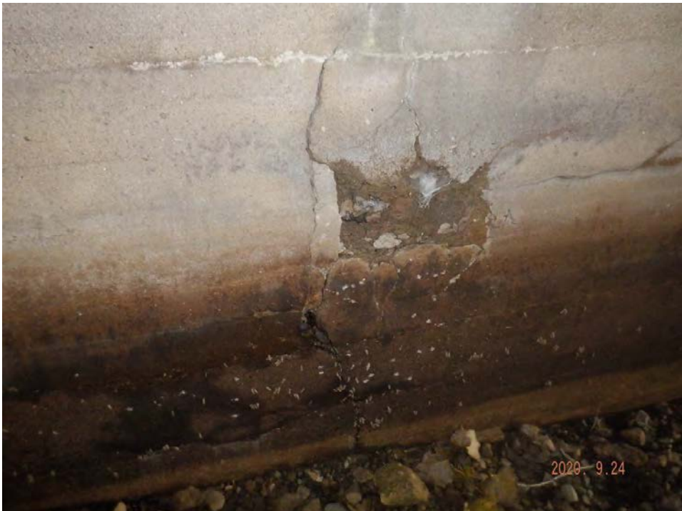
Spalling and delamination in east wall
