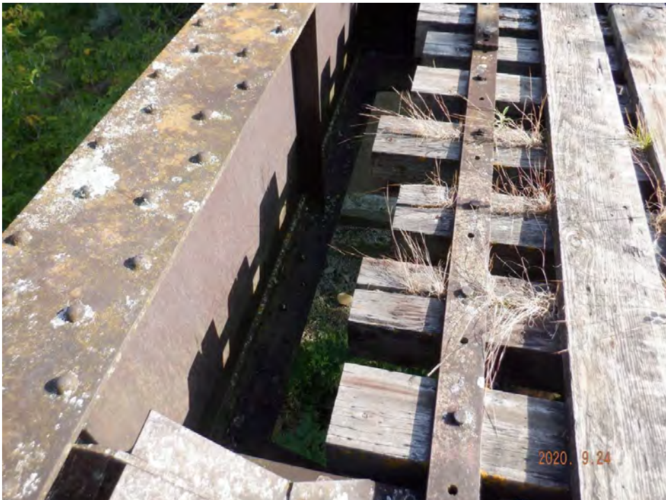
Gap between girder and deck edge
