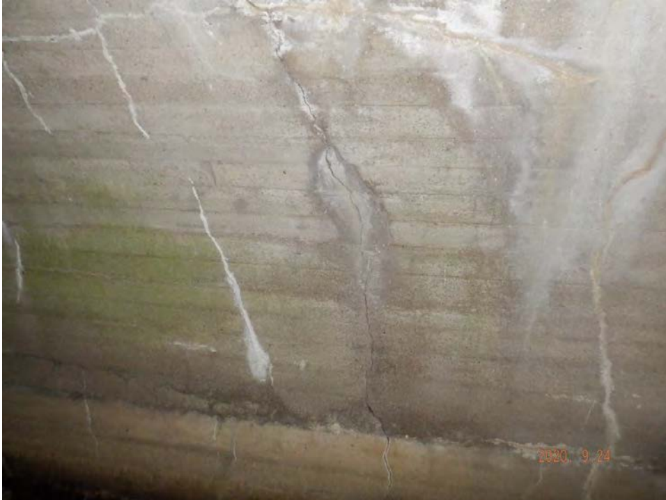
Cracking with efflorescence in west wall
