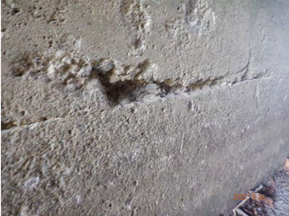
Honeycombing in east wall
