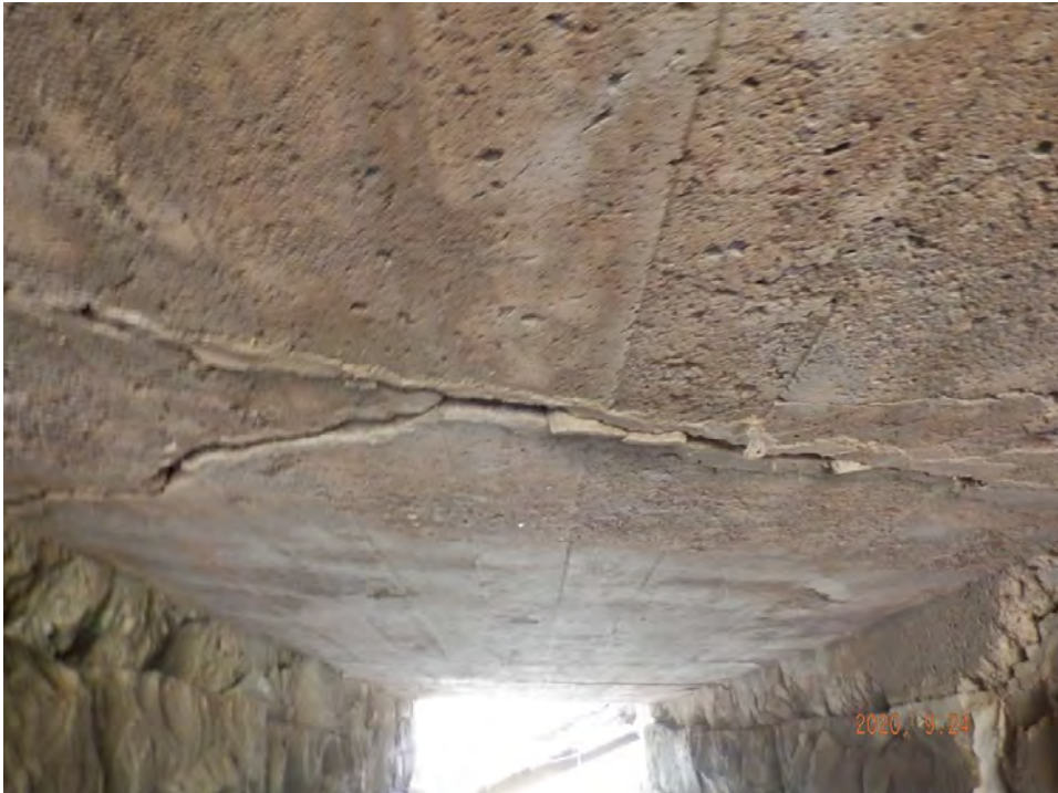
Cracking in soffit
