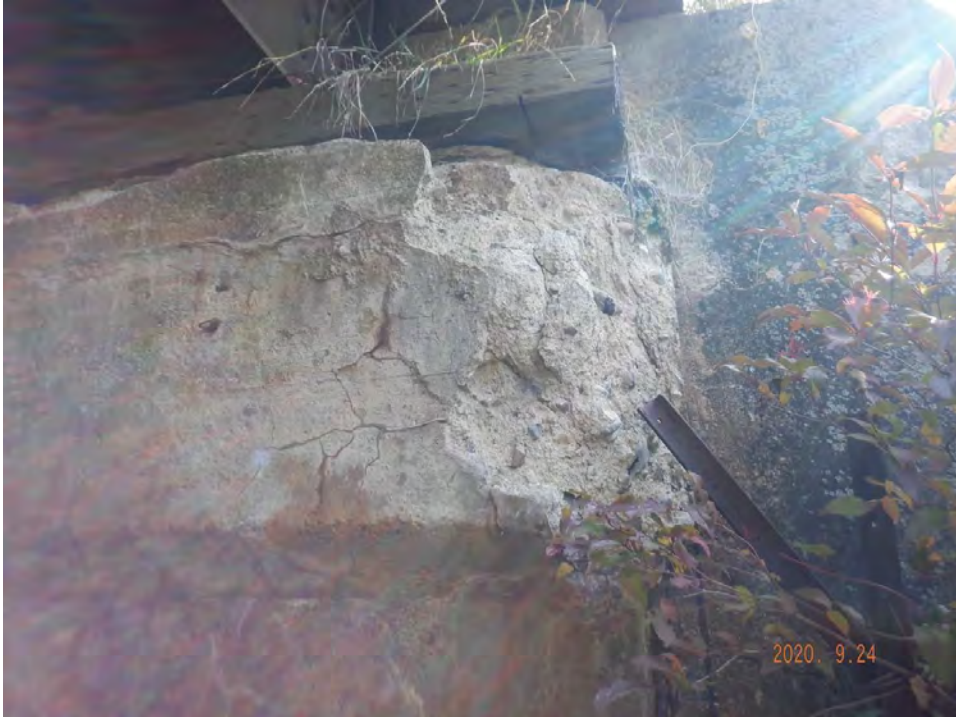
Disintegration in south end of east abutment
