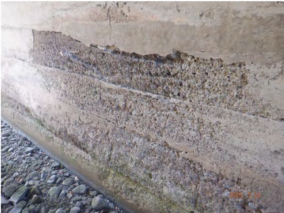
Moderate scaling in wall
