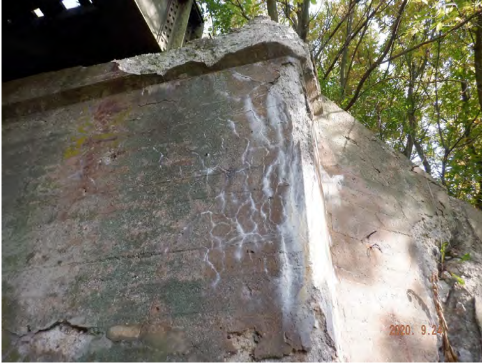
Cracking with efflorescence in southeast abutment
