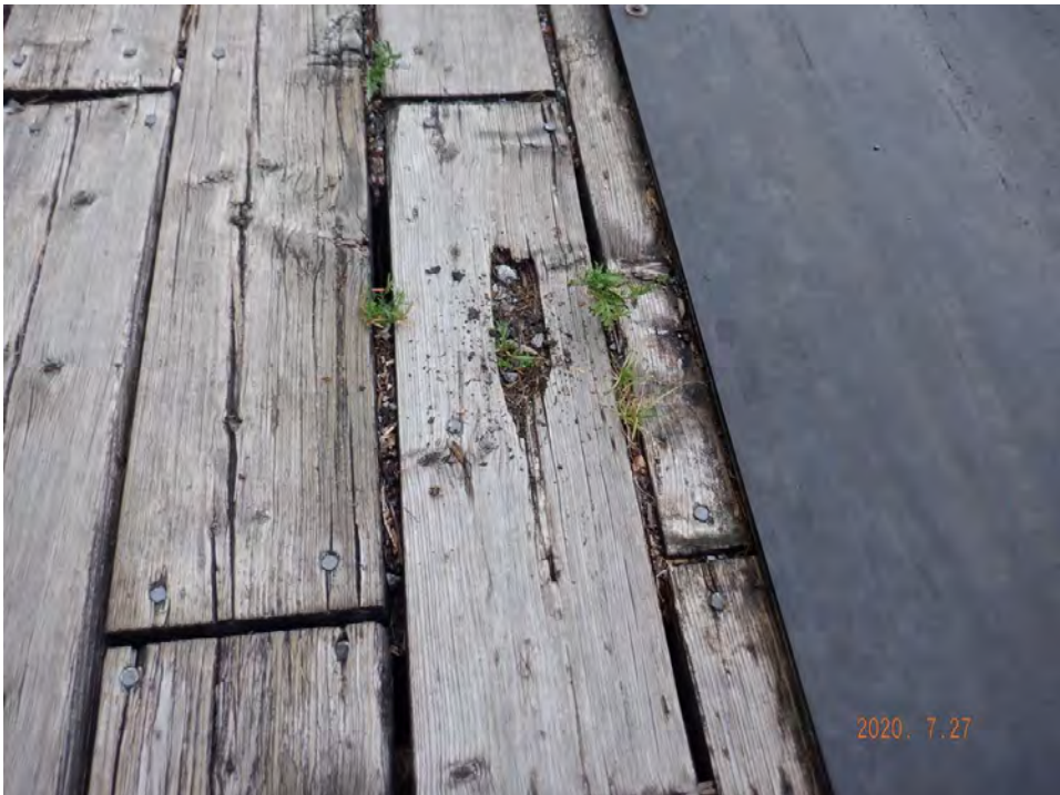
Rot in deck boards
