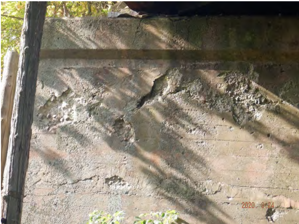
Disintegration in northwest abutment wall
