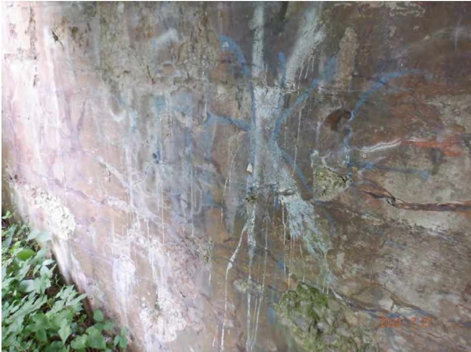
Light cracking and disintegration in west abutment wall
