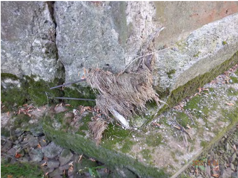
Spall in northeast footing
