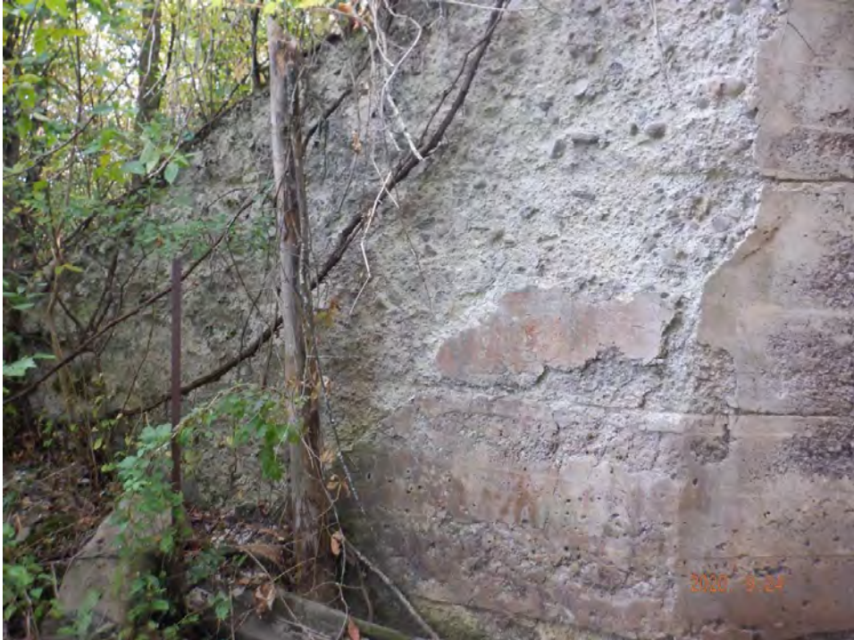
Severe disintegration in northeast wingwall
