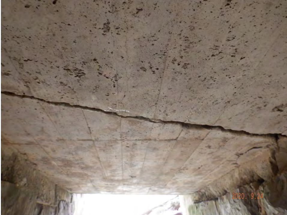
Wide crack in soffit
