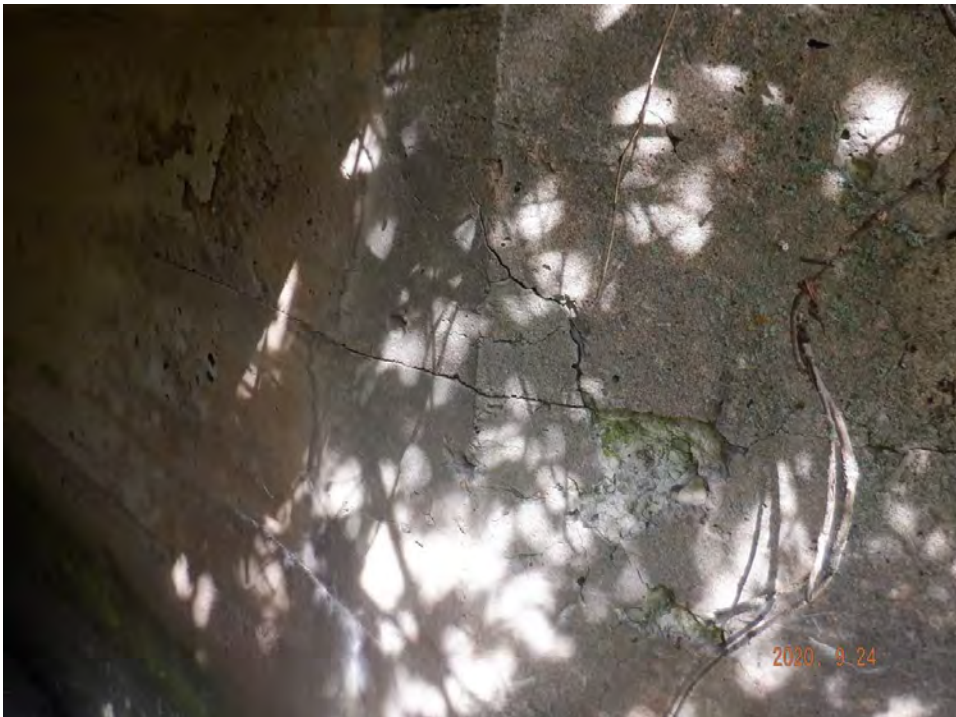
Cracking in southeast
