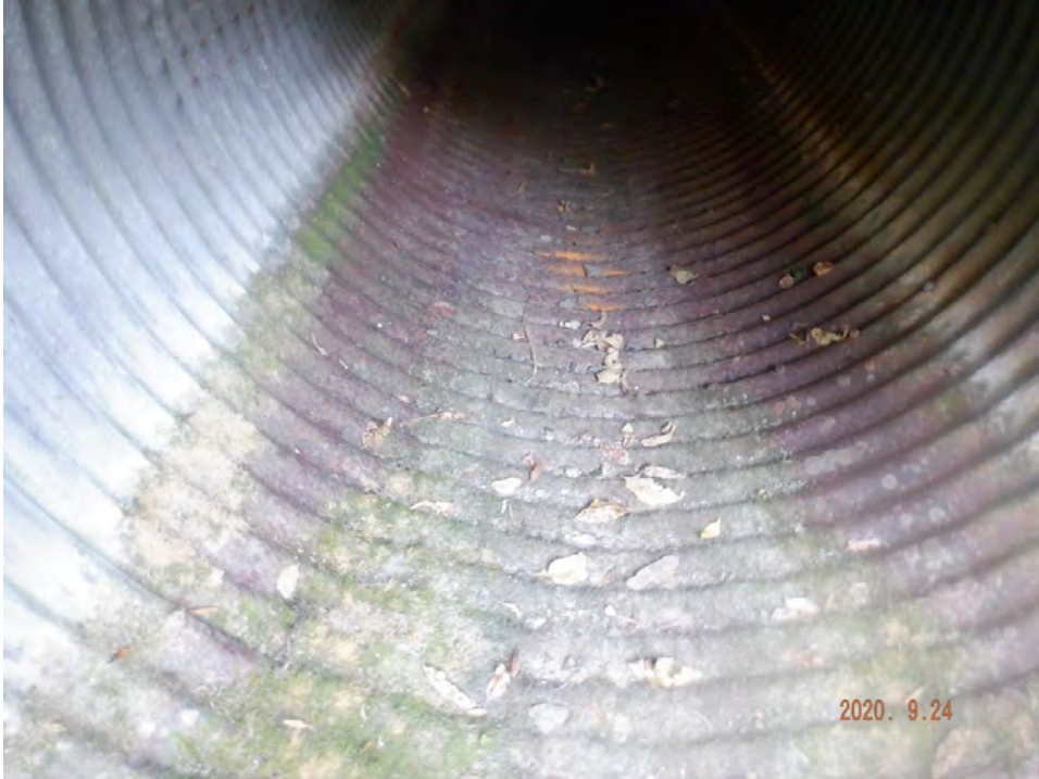
Typical corrosion in culvert floor
