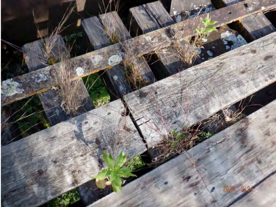
Rot and vegetation growth in railway ties
