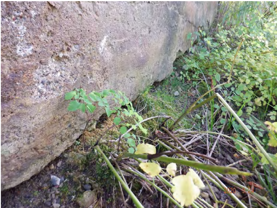
Erosion at base of east abutment wall
