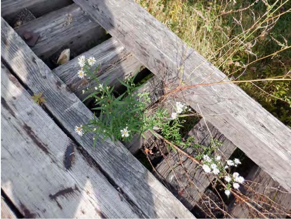
Vegetation growing in railway tie
