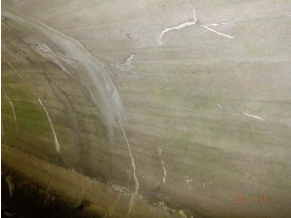
Cracking with efflorescence in west wall
