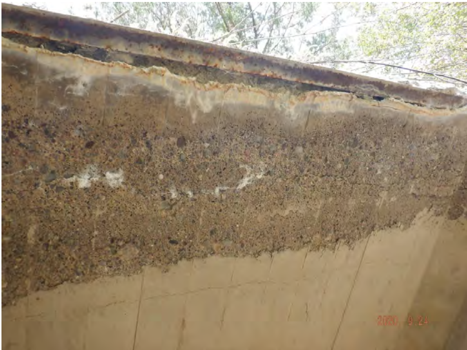
Scaling and disintegration in soffit end
