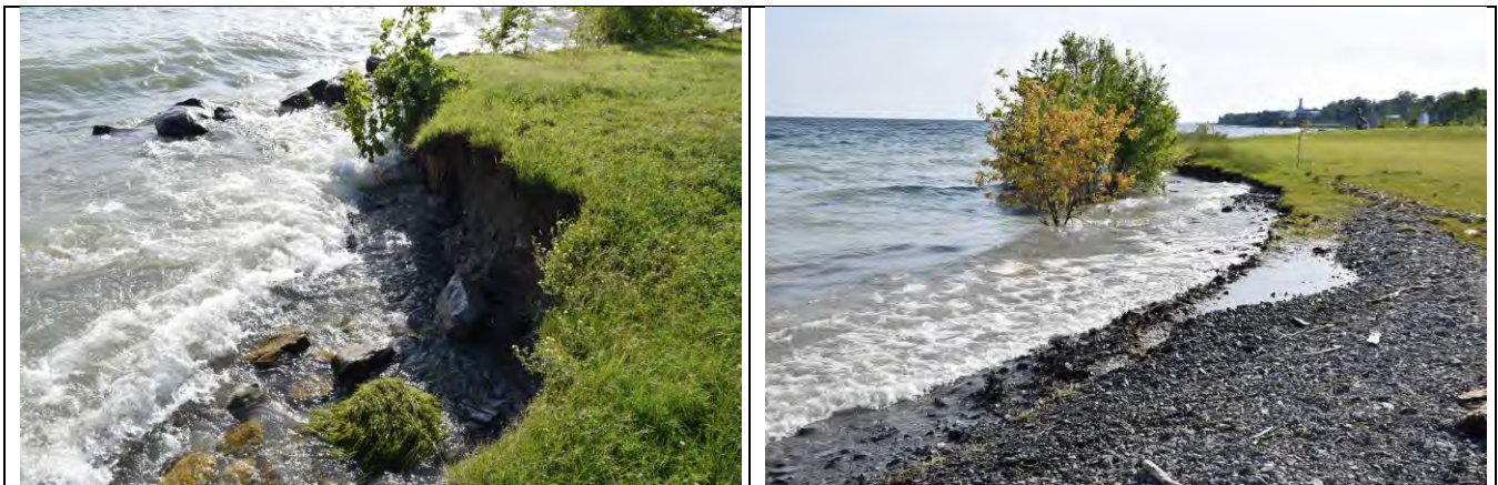
Figure 12 Shoreline erosion at Kingston’s Breakwater Park, June 2017
