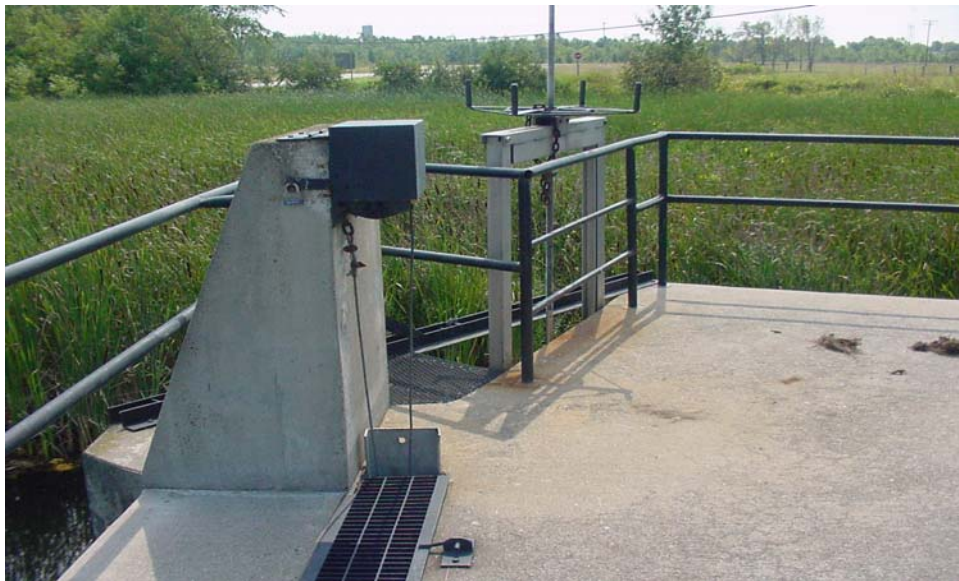
PHOTO WIL-15: LOW FLOW (GATE) VALVE OPERATOR
