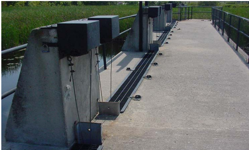
PHOTO WIL-14: WINCH PEDESTALS, GAIN COVERS, DECK, HANDRAIL WITH WIRE MESH (DOWNSTREAM SIDE ONLY)
