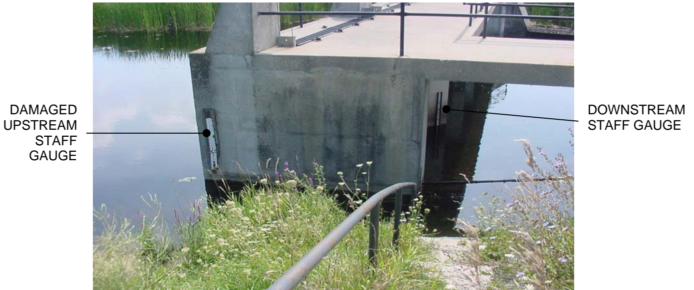
PHOTO WIL-09: STAIRS AND STAFF GAUGES
