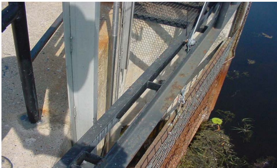
PHOTO WIL-16: TRASH RACK AT LOW FLOW VALVE
