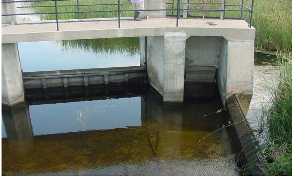
PHOTO WIL-11: LOW FLOW (GATE) VALVE (DOWNSTREAM VIEW)
