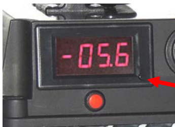
Figure 2 Amp meter showing discharge from an outlet socket
