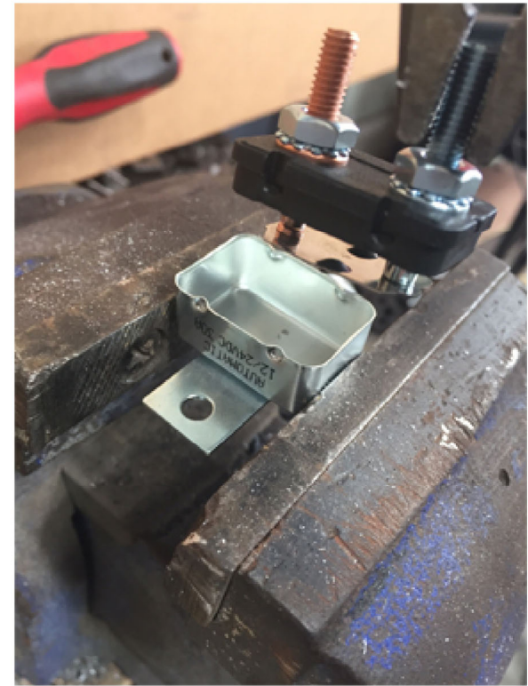
Once removed, you can install this into the base of the circuit breaker within your battery box
