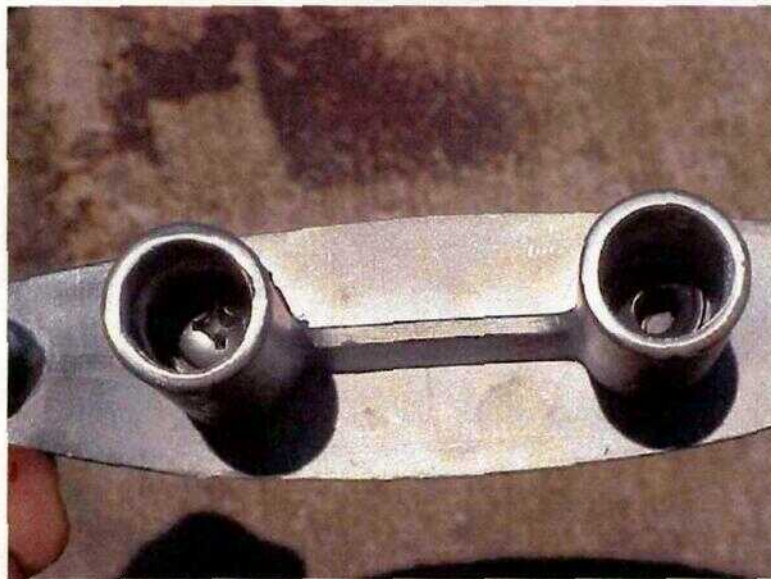
Figure 2. Close-up showing typical failure of Phillips cleat-retaining screw head breaking off. Note the absence of the Phillips head in the right side sleeve.
