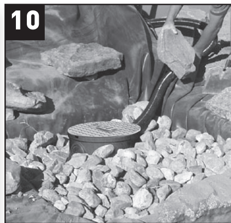
Fill basin with remaining gravel. Decorative gravel or smooth beach pebble can be added for the last few inches for a more finished appearance.
