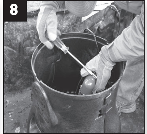
Attach hose to plumbing kit. Tighten hose clamp
