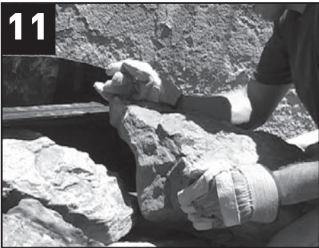
Use rock work and backfill to hide the Waterfall Weir and blend the new water feature into surrounding landscape.
