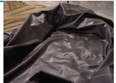
The liner covers the stream bed and goes through the area where the spillway will sit.
