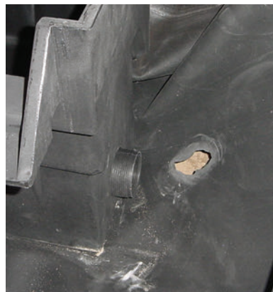
Hold bulkhead up to spillway and cut hole in liner just smaller than bulkhead.
