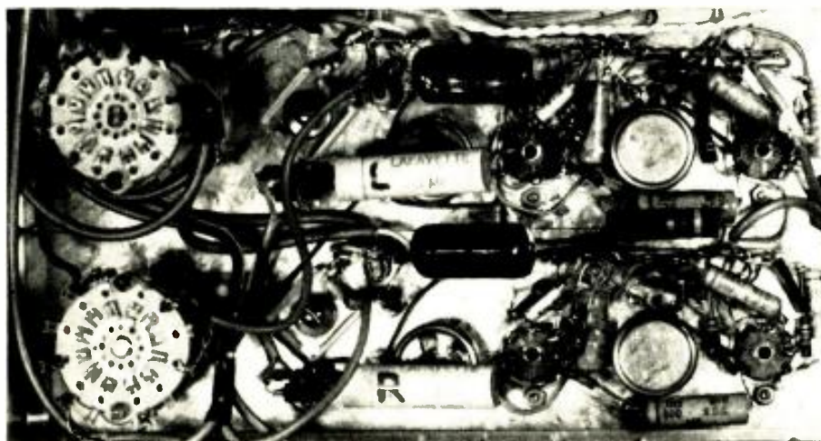
Inside view of the tightly wired recording preamps. Minimum lead lengths were used.
