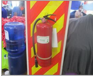
Photo of fire safety equipment Fire extinguisher.JPG
