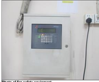
Photo of fire safety equipment Fire control pannel.JPG
