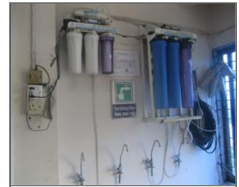
Photo of the sanitary facilities Drinking water point.JPG
