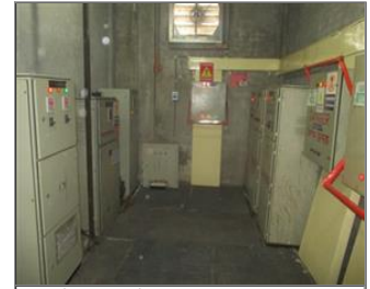
Photo of the inside of the main production hall Substation.JPG
