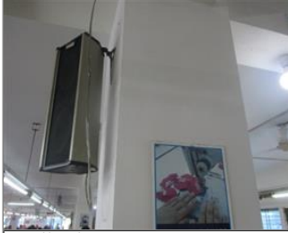
Photo of fire safety equipment PA system.JPG
