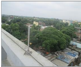
Photo of fire safety equipment Lightning arrester.JPG
