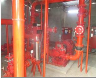
Photo of fire safety equipment Pump house.JPG
