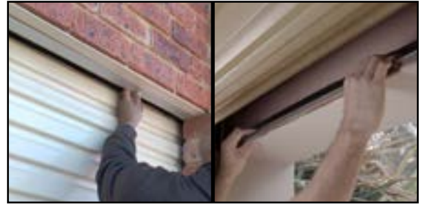
Exposed on lintel opening
