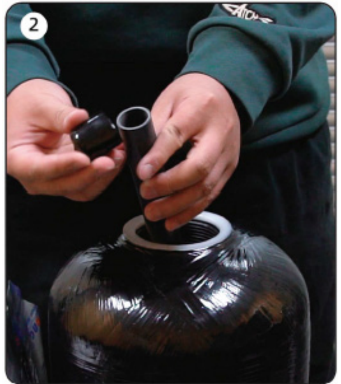
Connect plastic cap to the riser tube and put it in centre of the tank
