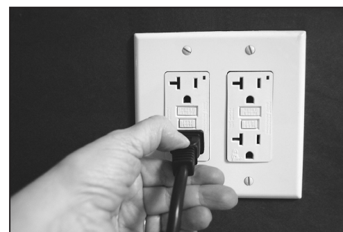
Test outlet with another appliance, and test the Electric cord in another outlet.
