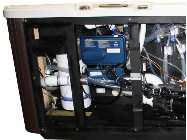
Equipment access is below the topside control panel.
