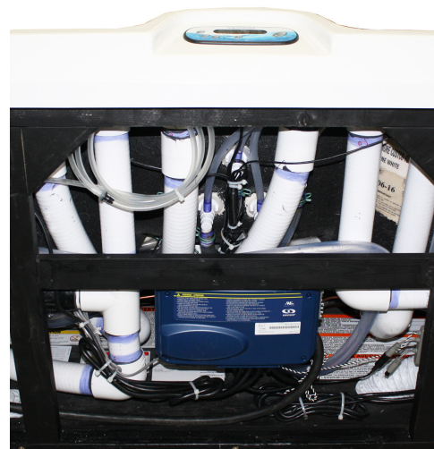
Equipment access is below the topside control panel.
