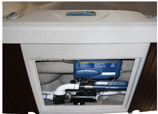
Equipment access is below the topside control panel.
