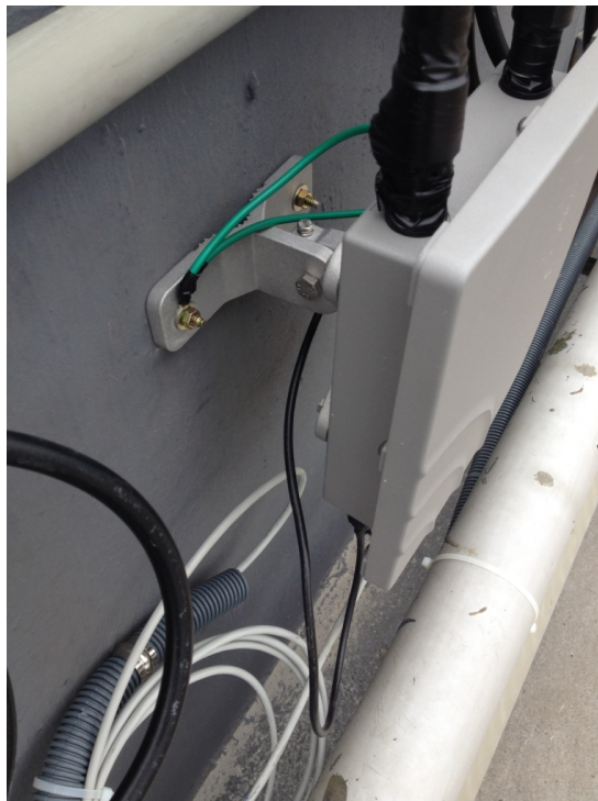
Figure 31 Lightning Protections and Grounding Equipment – Image 2
