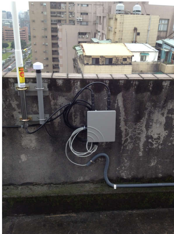
Figure 32 6 PVC cable protection hose
