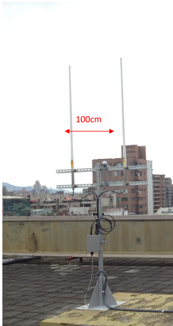
Figure 33 Actual View of a Base-mount Installation
