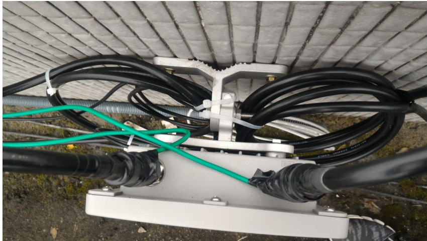
Figure 30 Lightning Protections and Grounding Equipment – Image 1
