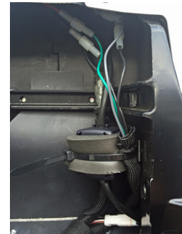
Figure 18. Signal wires with ferrite
