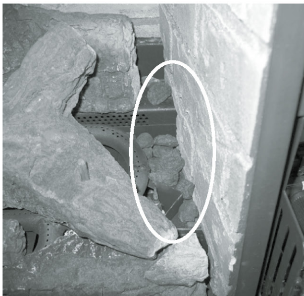
Right side of Burner
