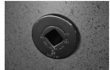
Key Valve Assembly (Outside View)
