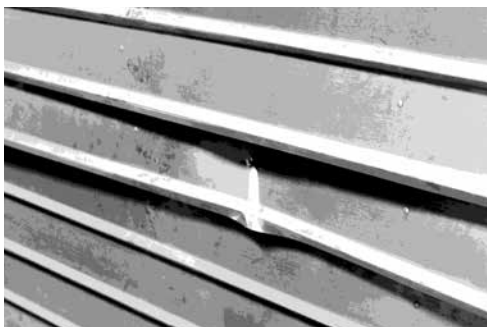
Fig.1 - Damaged louver vane needs replacing
