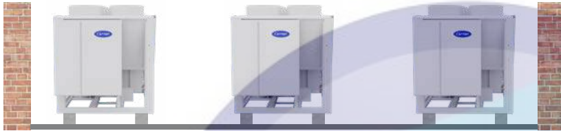
Chillers side by side with brick walls at the end
