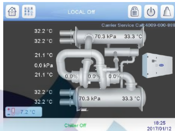
Fig. 26 Chiller Start/Stop Icon
