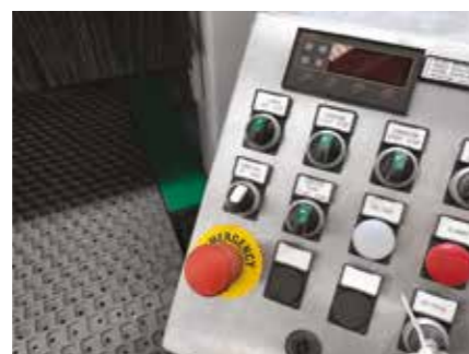
Control by PLC
