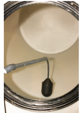
Pre Installed Float Switch
