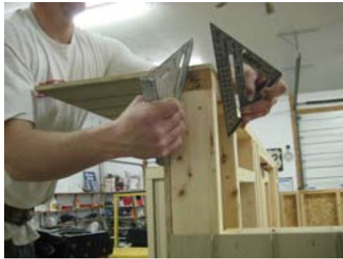
Install LP Smart siding strips on the front wall as shown. Keep flush on inside and secure with 1 1/4" zinc screws going into 2x4 top plate.
