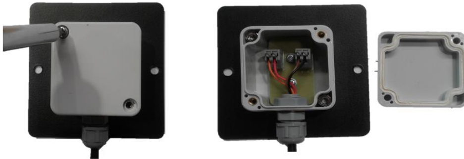
Opening the back of the wallswitch
