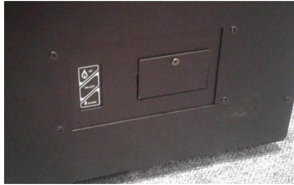
Photo 5: Receiver batteries containers
