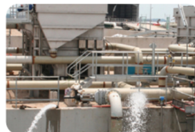
Water Treatment Facility
