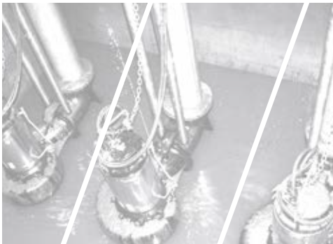
Wastewater Transport and Treatment
