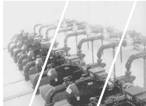
Boosting and Distribution of surface water
