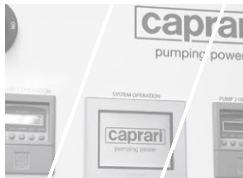
Pump Control Technology
