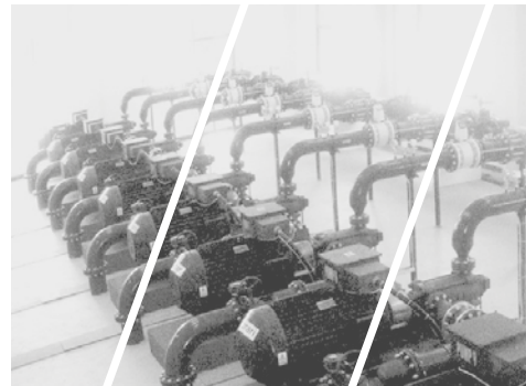
Boosting and Distribution of surface water
