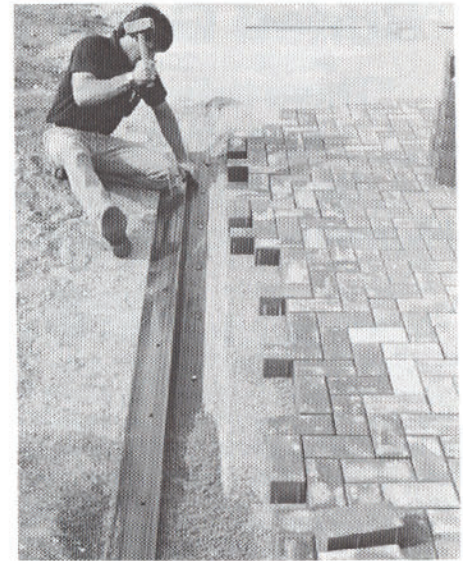
Jeff Clapp of Pave Tech installs PAVE EDGE INDUSTRIAL on the one open side.
