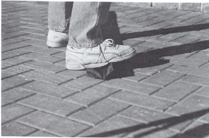
Bric Edge® cannot even withstand foot pressure without bending.
