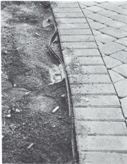
Installer failure, not PAVE EDGE
