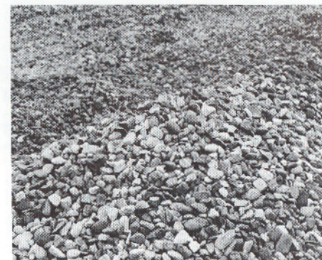
This type of aggregate is unacceptable for base
