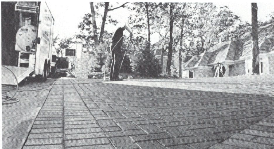
Sealer should always be applied starting at the highest elevation of the pavement, working side to side to the bottom of the slope.
