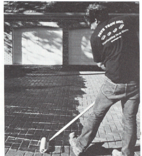
PAVE TECH recommends a powered roller type of application for sealing, but either high or low pressure sprayers will do the job.
