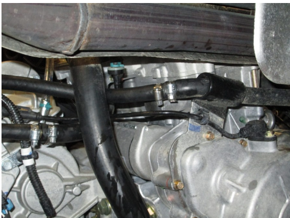
23. Trim line as needed and fasten this connection with the 3/8" barbed union and (2)#6 hose clamps.
