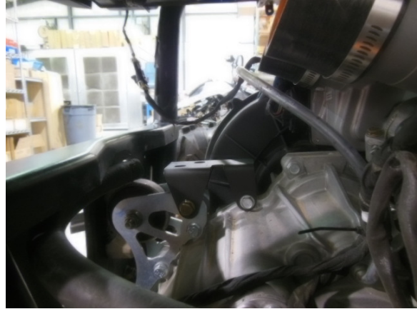
14. Install air box transmission mount bracket using stock bolts and steel spacer from stock air box. Leave bolts loose so air box can be adjusted later.
