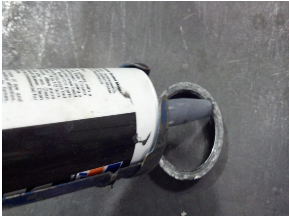
21. Remove small exhaust donut and run a bead of silicone on inside and seal to the end of the pipe.
