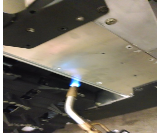
20. Using a torch or heat gun. Heat up the access panel to break the glue bond. Note it may require prying to break loose. (use caution to prevent a fire)
