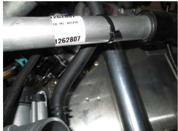
30. Route longer turbo coolant hose to throttle body as shown, cut to length and connect to throttle bodies.
