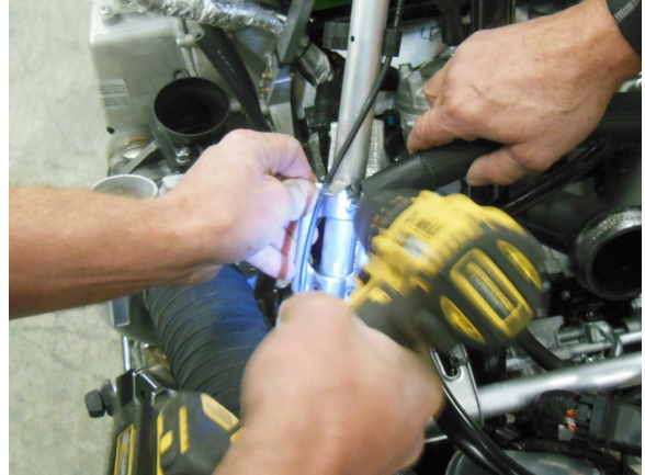
56. Drill out rivets holding mounting bracket to overstructure. Use a vacuum to ensure metal shavings don't get into engine systems
