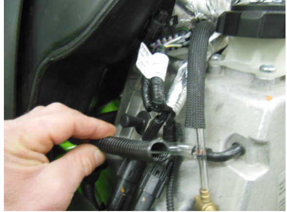
14. Pull back the tubing protector to expose the factory return oil line. Cut the clamp and remove the line from tank.
