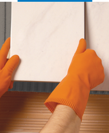
Installation of ceramic tiles on a wall using Mapeset with high thixotropic properties
