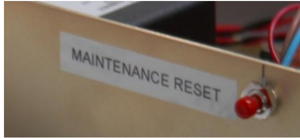
Figure 12 – MAINTENANCE RESET button
