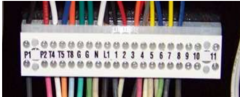
Terminal Strip inside main control Box
